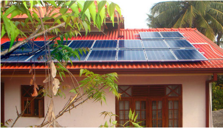
Location : Gampaha, Sri Lanka Power Generation : 580- 620 Units per month
