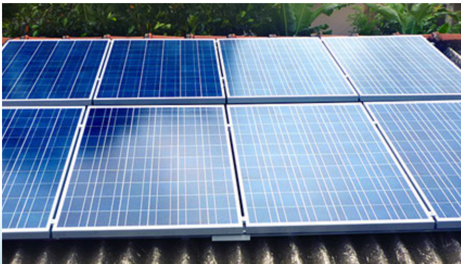
Location : Gampaha, Sri Lanka Power Generation : 240- 260 Units per month
